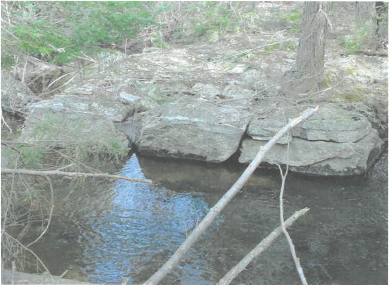
Rock Abutment where bridge and road were located photo taken Spring 2006
